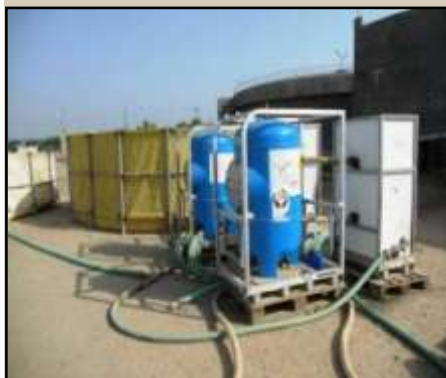
Water Treatment Unit installed in Ranjhan pur and Jacobabad
